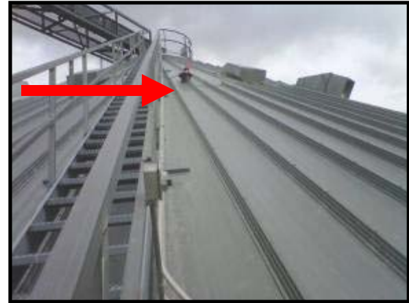
Scanner #1 mounted near the center of the bin, but away from the fill stream.
