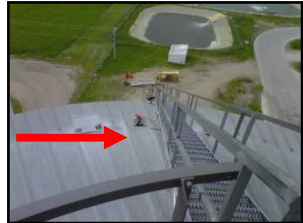
Scanner #2 mounted 1/6 from the outer perimeter of the bin.
